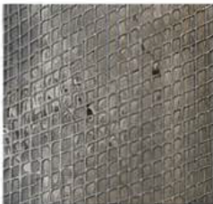
UV DEGRADATION AND BRITTLINESS
